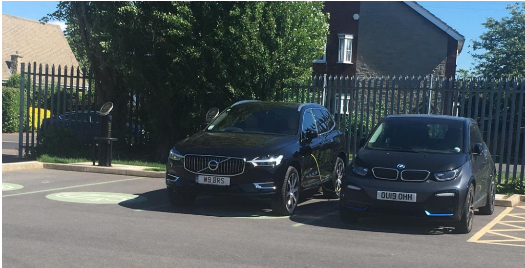
EV charging points at Doncaster office
